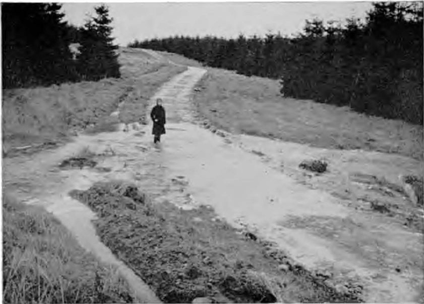
Plate 23. Blankenburgs: A flood on a forest road, due to the use of too small a culvert.
