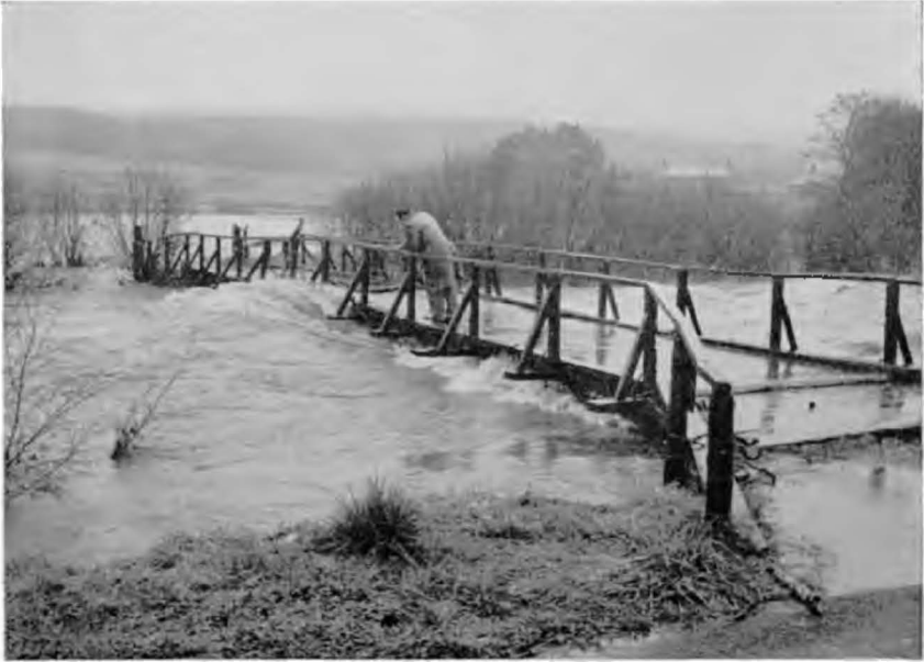
Plate 22. Blankenburgs: Waterways: A forest road bridge in danger, because the waterway is too small.
