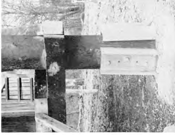
Plate 9. Packwood, Fire Tower: Details of the basal support of one main pole of the new Emery Down Tower.
