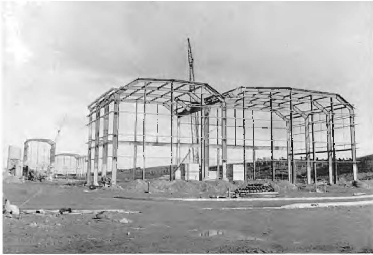
PLATE 15: Progress in the erection of the Thames Board integrated pulp and board mill at Workington, Cumberland. This part of the building will be the machine house and will be some 765 feet in length.
