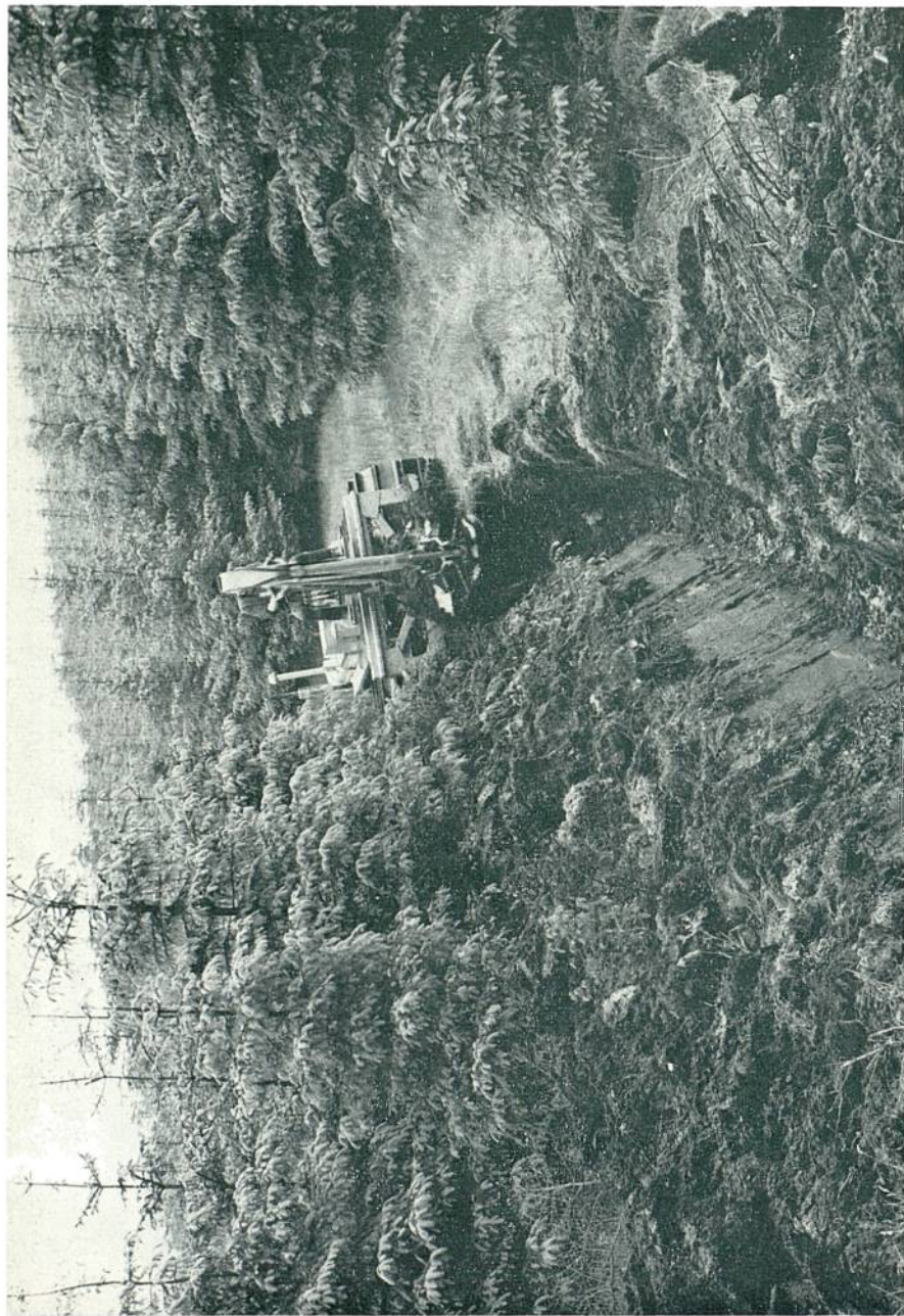
PLATE 6. Digging a deep drain in Carron Valley Forest, Stirlingshire, using a back-acter excavator powered by a crawler tractor. Deep drainage of this heavy clay soil is designed to bring spruce plantations out of "check", and raise their Production Class.
