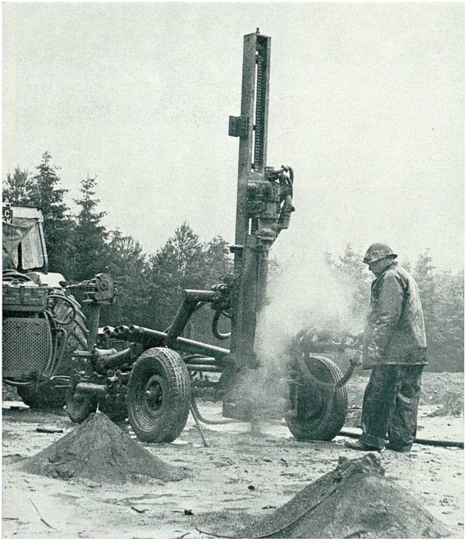
Plate 8 A Holman Universal Drilling Rig drilling a planned blasting pattern to provide fragmented rock of a size suitable for crushing to road stone at Brechfa Forest, Dyfed, South Wales.
