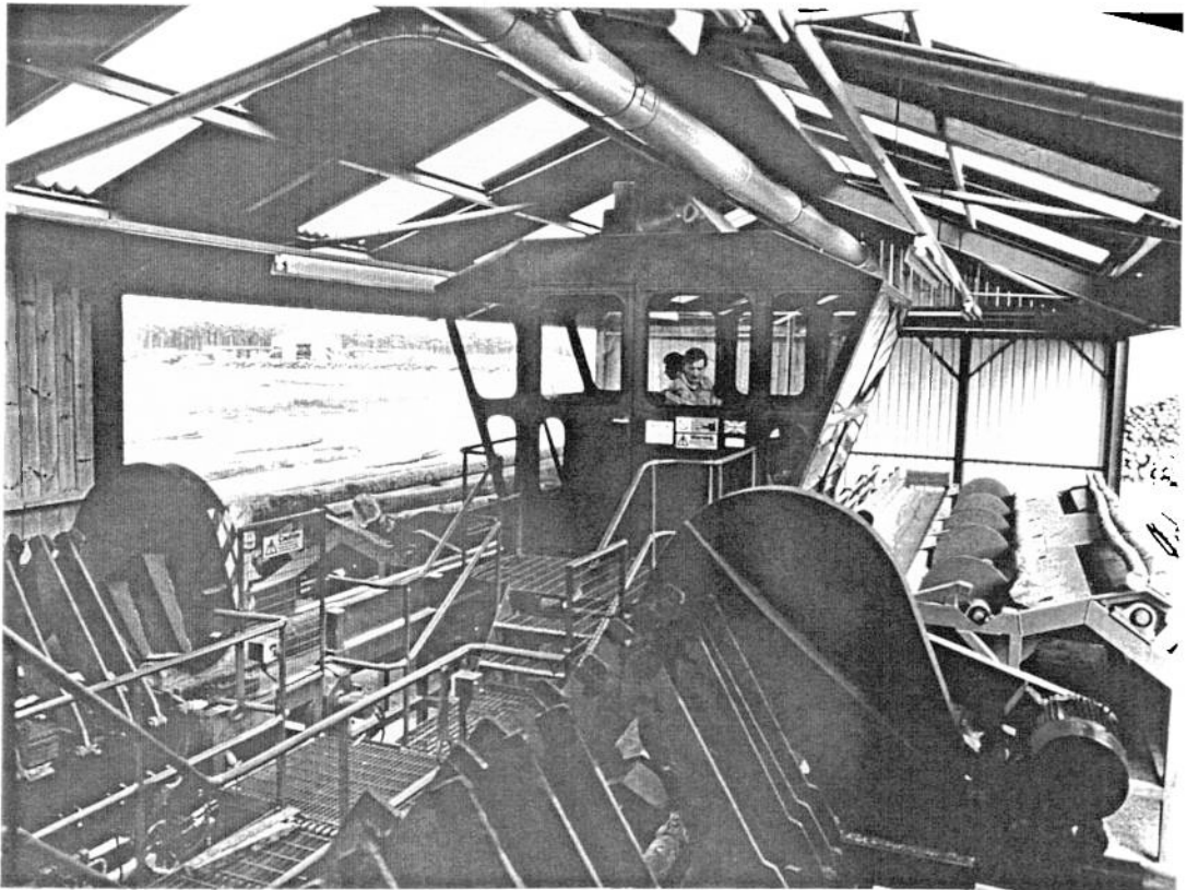
Plate 36. Control cabin No 1 & 2 crosscut stations with steps and circular crosscut saws. Note singling device between infeed deck and sawfeed conveyor
