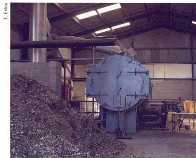
PLATE 59 Wood chips from urban trees being used to fuel a boiler heating 2 acres of glasshouses; Leeds City Council.
