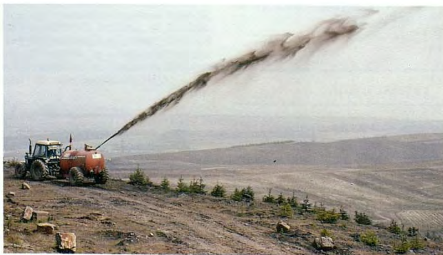
Liquid sludge application to opencast coal spoils and Maesgwyn. The tanker is capable of delivering nearly 100 \text{ l s}^{-1} over a distance of 100 m. Treated spoil in foreground. (39424)
