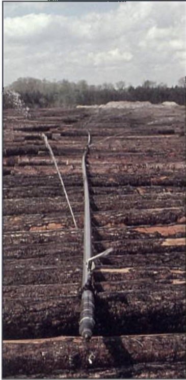
Plate 4 Sprinkler system in action on the log stack. (38789)
