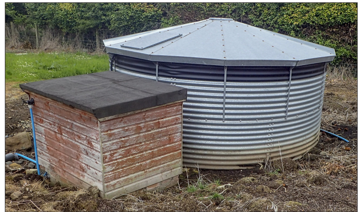
Covered borehole water storage tank.
