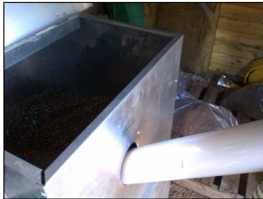
Figure 11 – Boiler pellet hopper
