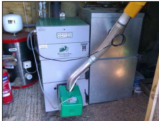
Figure 10 – 20kW Woodpecker boiler
