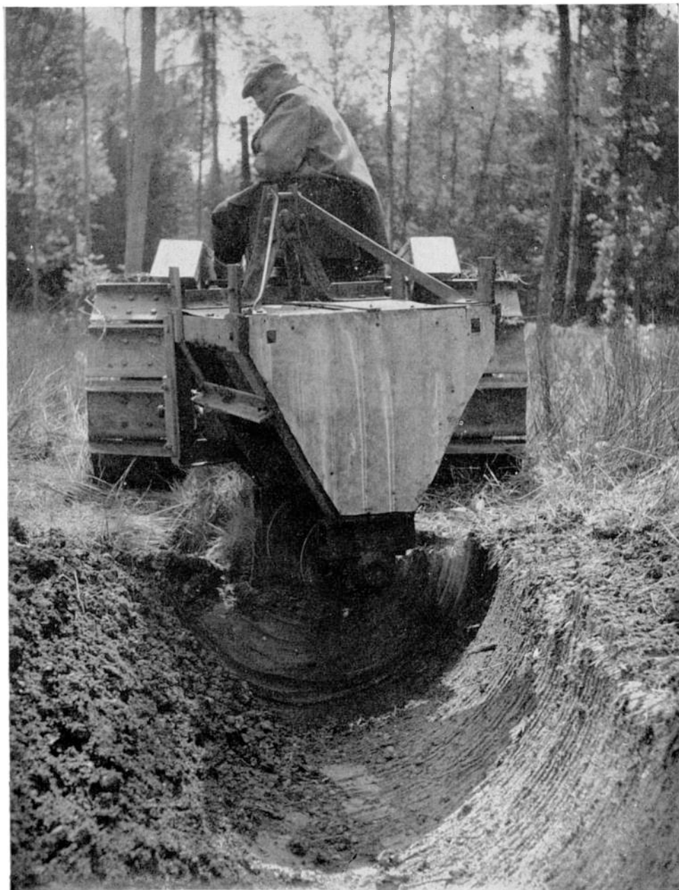
PLATE 14. Shaw: Machinery Research: A prototype of the new flail type drain cleaning machine developed by the Forestry Commission for cleaning surface drains to a depth of 18 inches.
