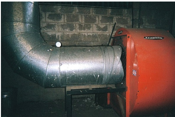
Hot air boiler
