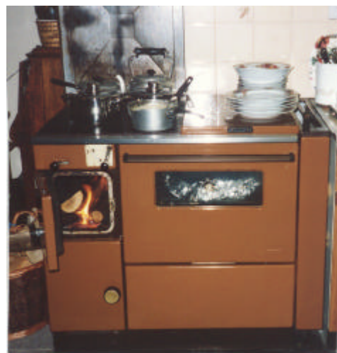
18 kW log fuelled cooker/boiler (small farmhouse) shown with loading door open
