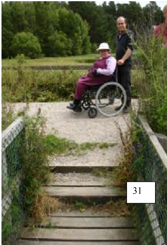
Fig 31: ramps required for bridge access.
