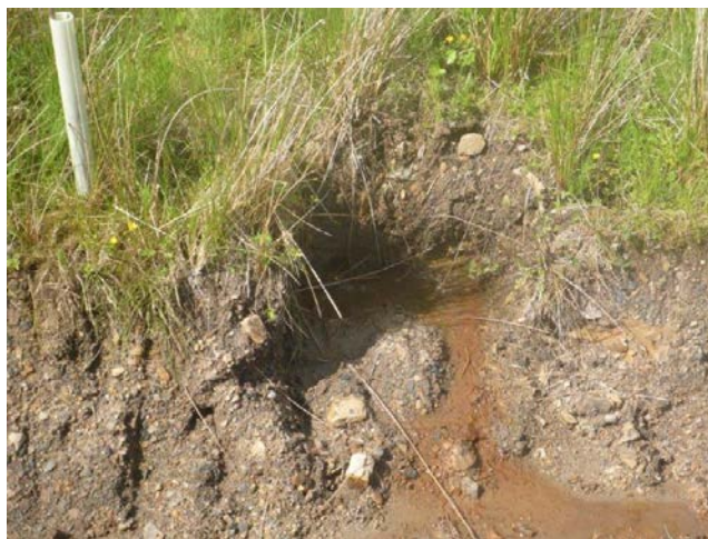
Drainage tap, September 2015
