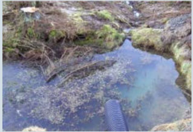
Figure 33b An example of a poorly designed silt trap: culvert aligned with outflow, promoting slip-streaming, while hanging inflow will generate turbulence and stir up sediment.
