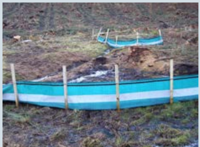
Figure 33f Use timber posts at a slight upslope angle to support longer lengths of geotextile barrier. Consecutive barriers, as shown here, may be needed to manage a sediment pollution incident.
