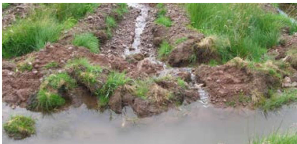
Figure 35 Heavy rainfall has resulted in water overspilling from a drain into a lower cultivation channel, causing erosion and turbid water discharging into a watercourse.
