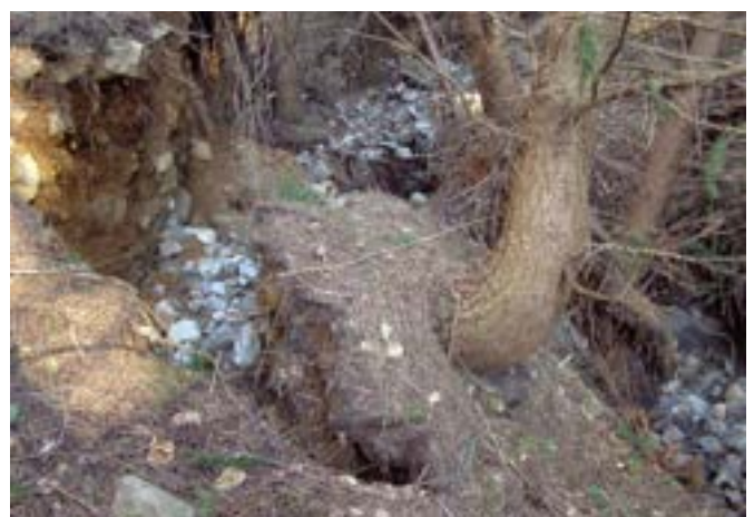
Figure 22 Seek hydrological advice on how to manage eroding gulleys, including how to remedy overloaded watercourses.
