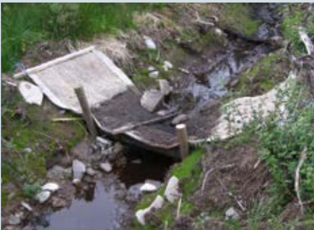
Figure 33c Coir matting can help trap fine and coarse sediment across a range of flows.
