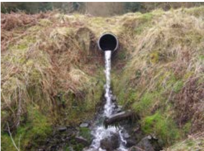
Figure 16 Hanging culverts should be avoided, especially in fish-bearing streams.
