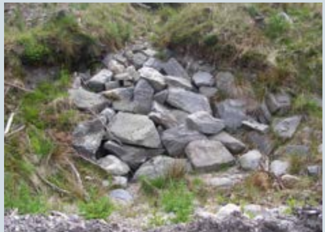
Figure 33d A collection of different sized stones can provide an effective drain-end sediment trap.
