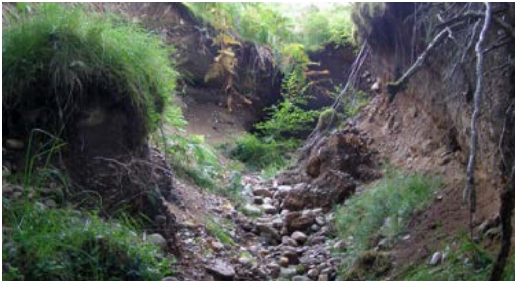
Figure 6 Excessive run-off has caused major erosion and gullying within this drain.
