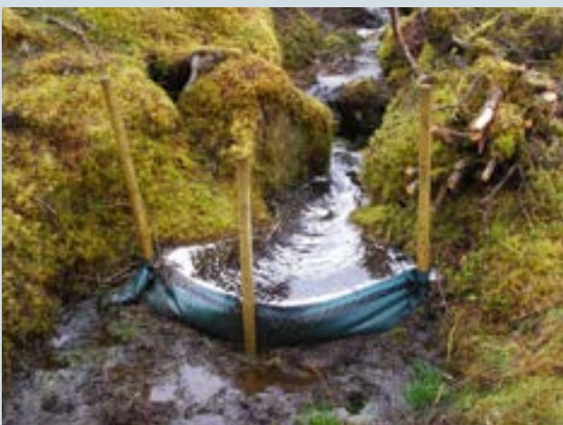
Figure 33e Terrain fabric can be used to create a small silt trap but is readily bypassed by significant flows.
