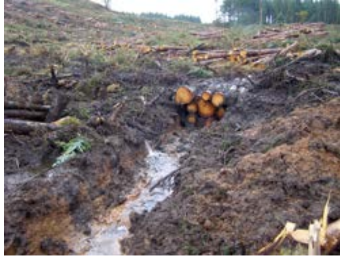
Figure 28 In this situation pipes need to be installed along with logs to prevent water backing up and causing site waterlogging and ground damage.
