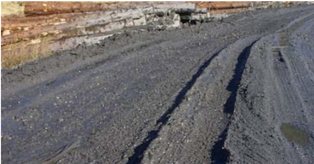
Figure 14 Damaged road surfaces can quickly degrade and cause pollution through sediment run-off.
