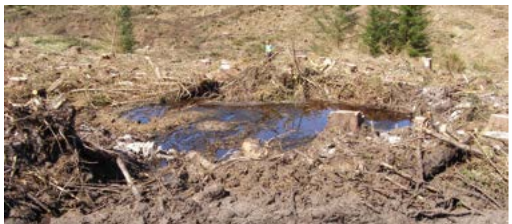
Figure 32 A brash bund can provide an effective filter for retaining sediment, providing run-off volumes do not exceed the capacity of the system.
